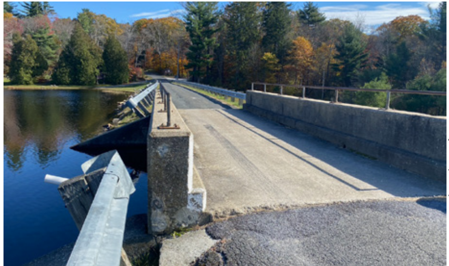
A guard rail on the roadway over the York Lake dam is failing.
