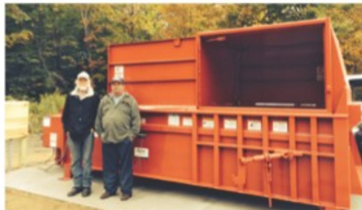
Once the single-stream compactor was lowered onto a new concrete slab, transfer station managers Alvin Stalker, left, and Bobby Litchfield took a proprietary interest. photos by Peter Schuyten
