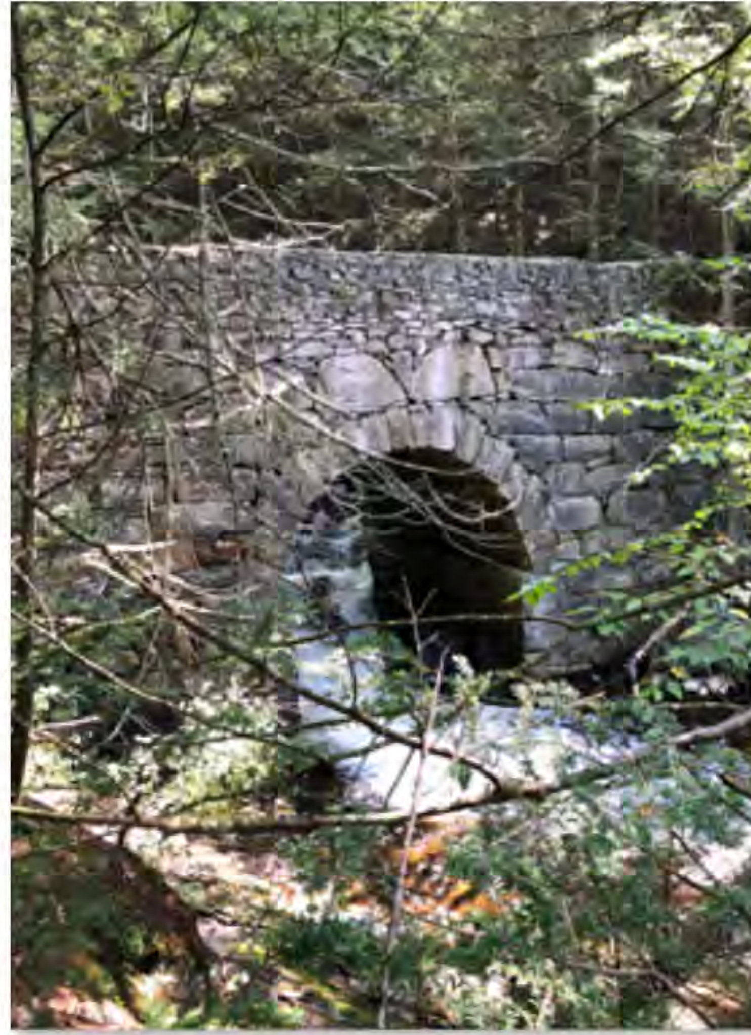
A view of the south facade of the Campbell's Falls Road bridge photo by John Schreiber
