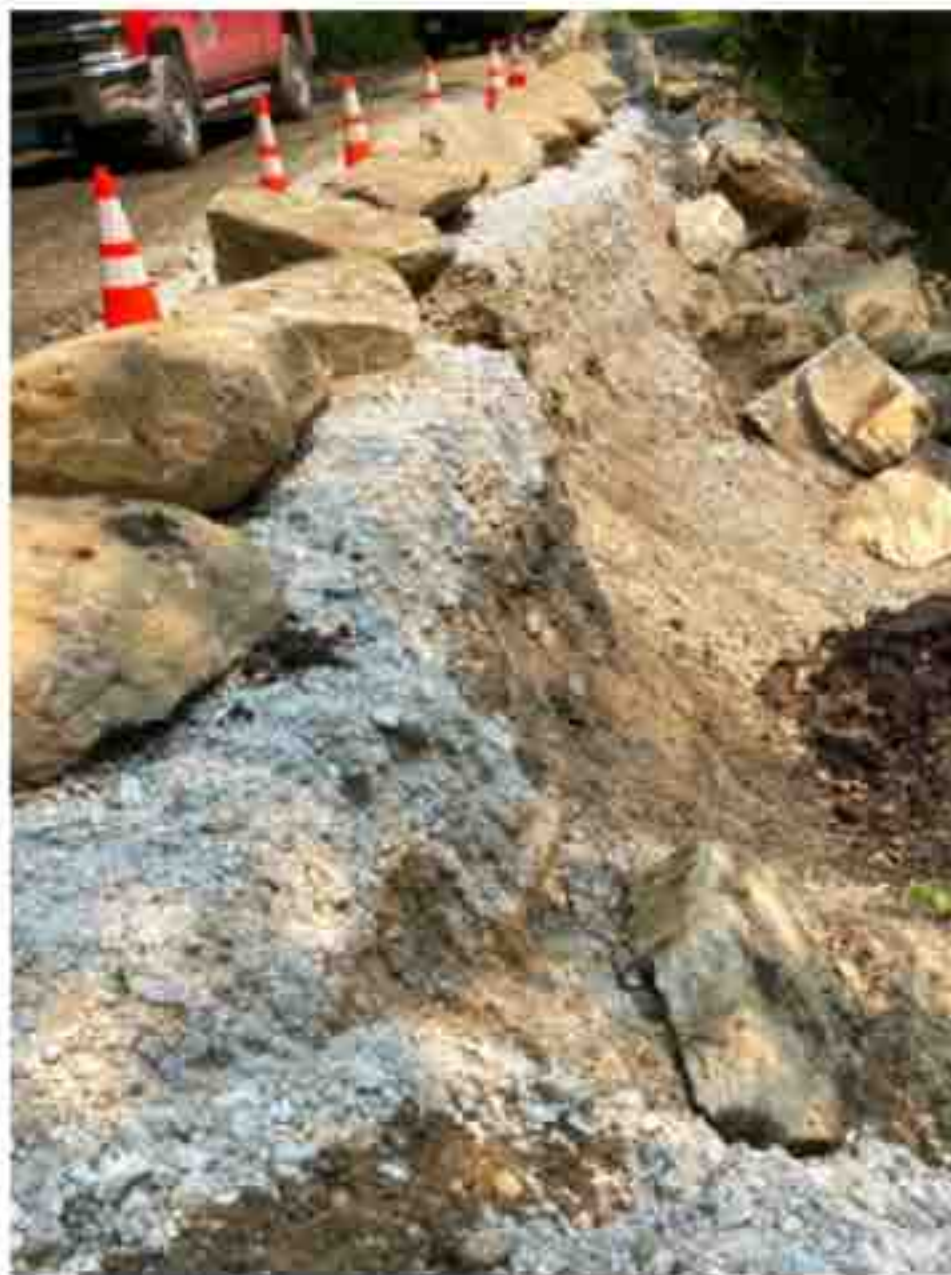
A section of Campbell Falls Road suffered a rain-induced collapse. photo by Chuck Loring
