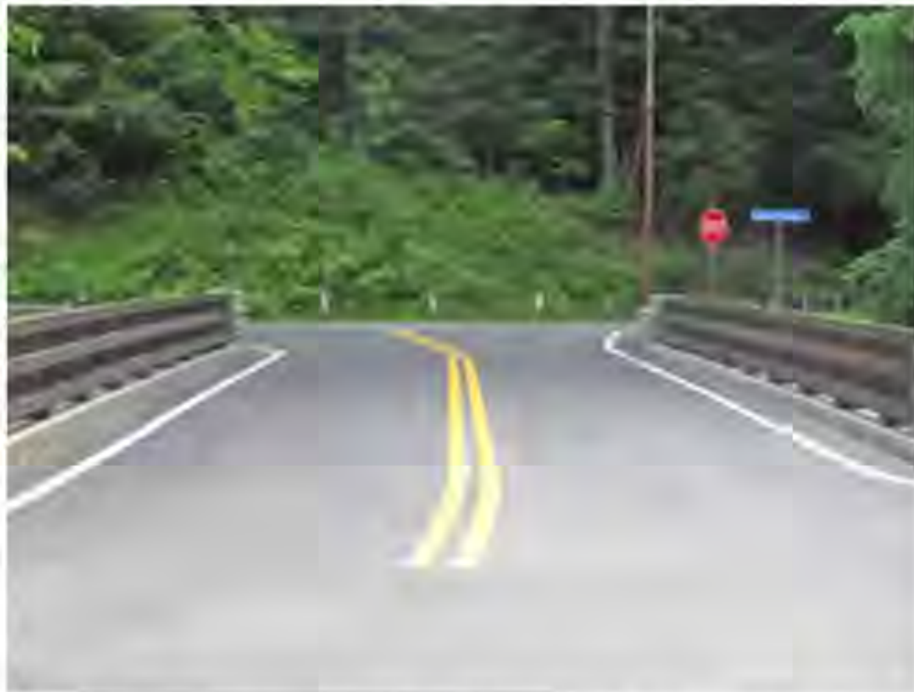
Closed for seven years, the Hadsell Street bridge was re-opened on June 11! photo by Joe Poindexter
