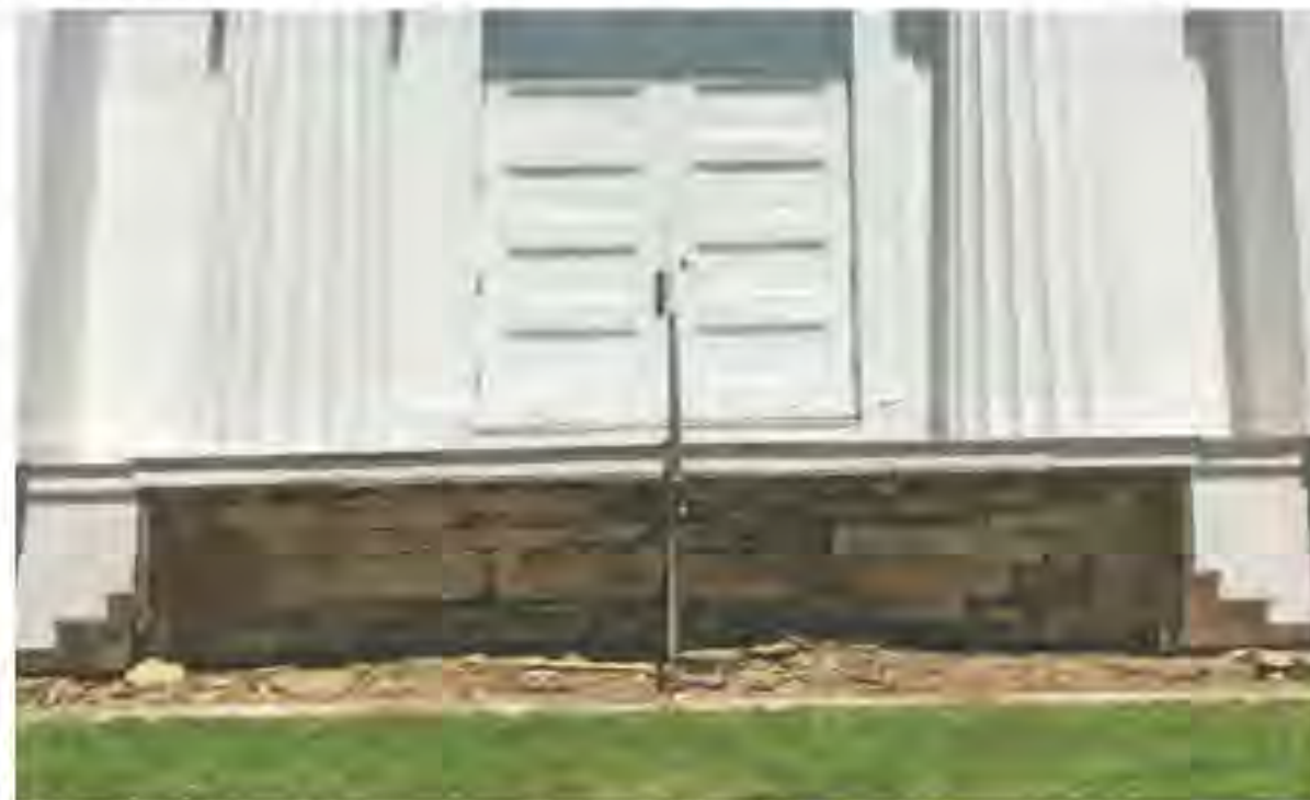
Removal and excavation of the existing steps revealed a crumbling foundation in need of reinforcement from a cement retaining wall.
