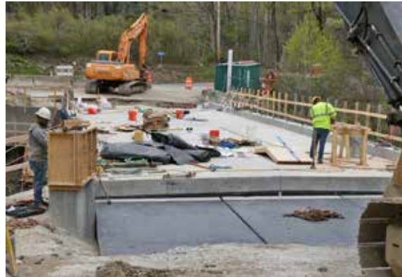
A month ago, the new span awaited connection ramps to Norfolk Road.
