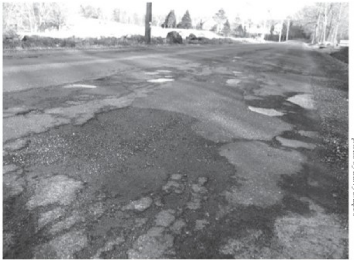
County Road potholes ...
