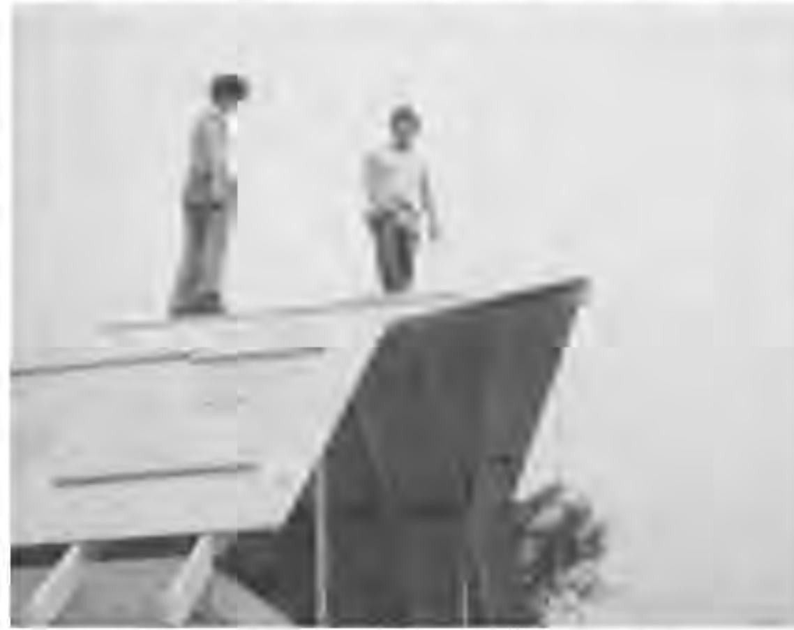
Leon and a son, Bruce, put a roof on the new house.
