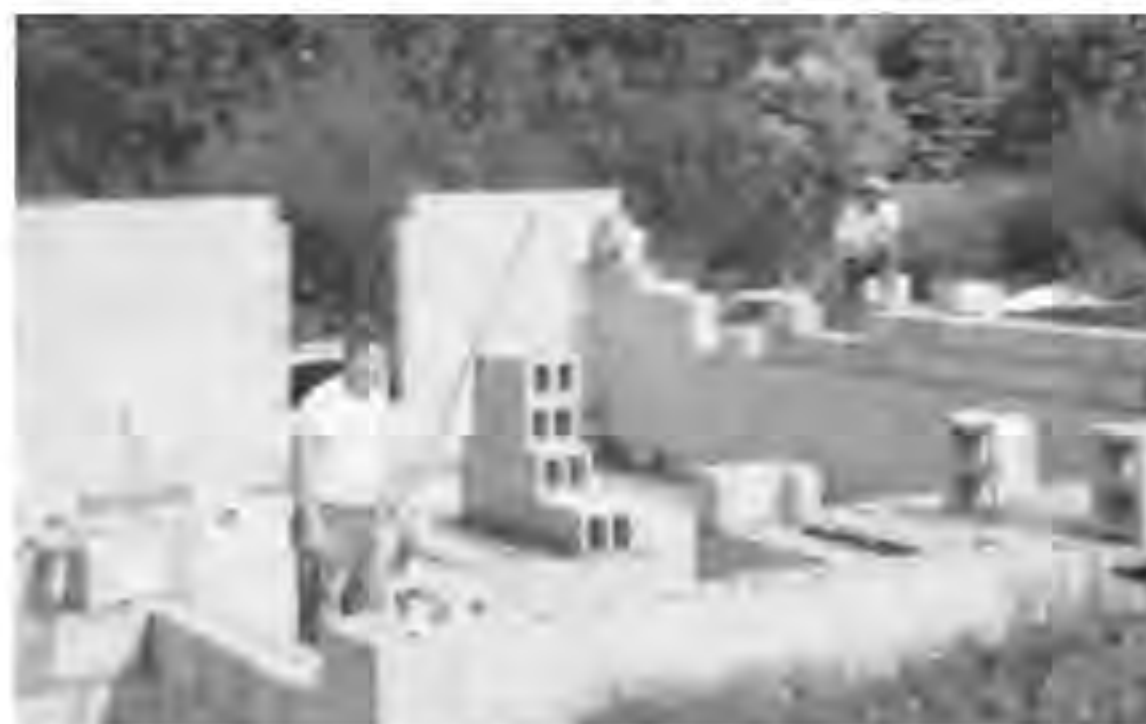
Leon, left, and George Denard built the foundation of the Eichstedt house.
